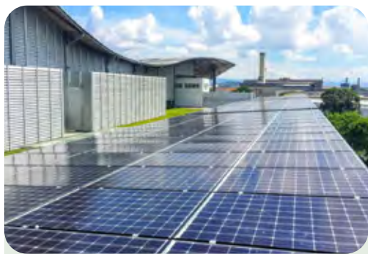
Solar panel at UOM
