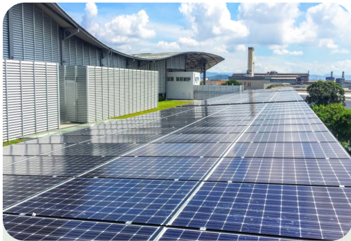
Solar panel at UOM
